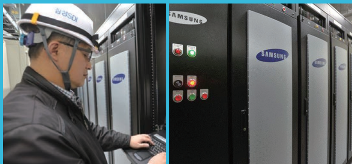
UES installed at Uiwang Site
