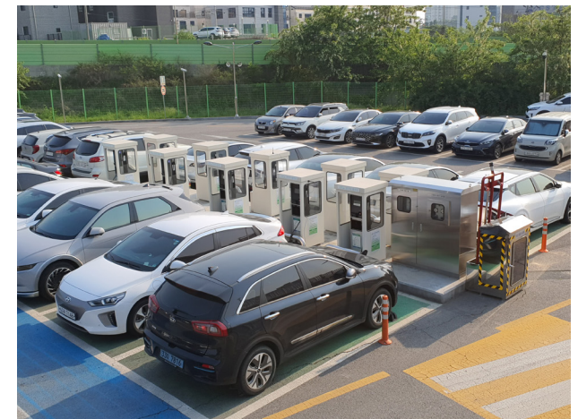
EV charging area at our Giheung worksite
