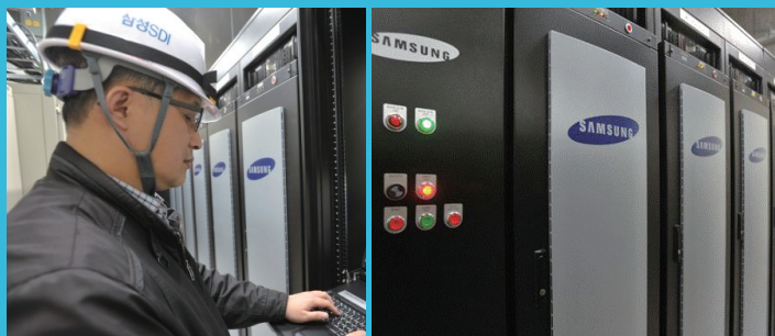
UES installed at Uiwang Site
