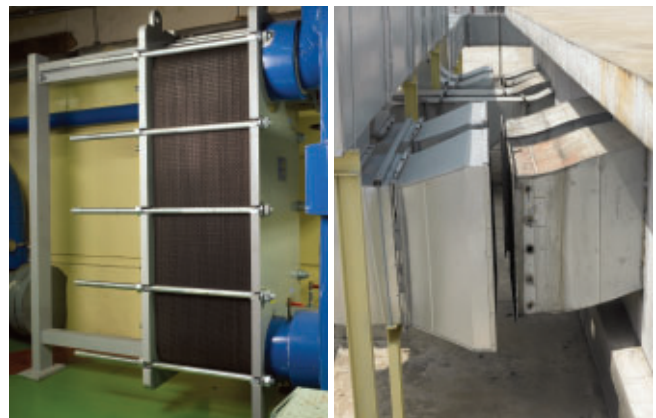
| Energy saving: Heat exchanger(Busan) and Waste heat recycling facilities(Cheonan) |
